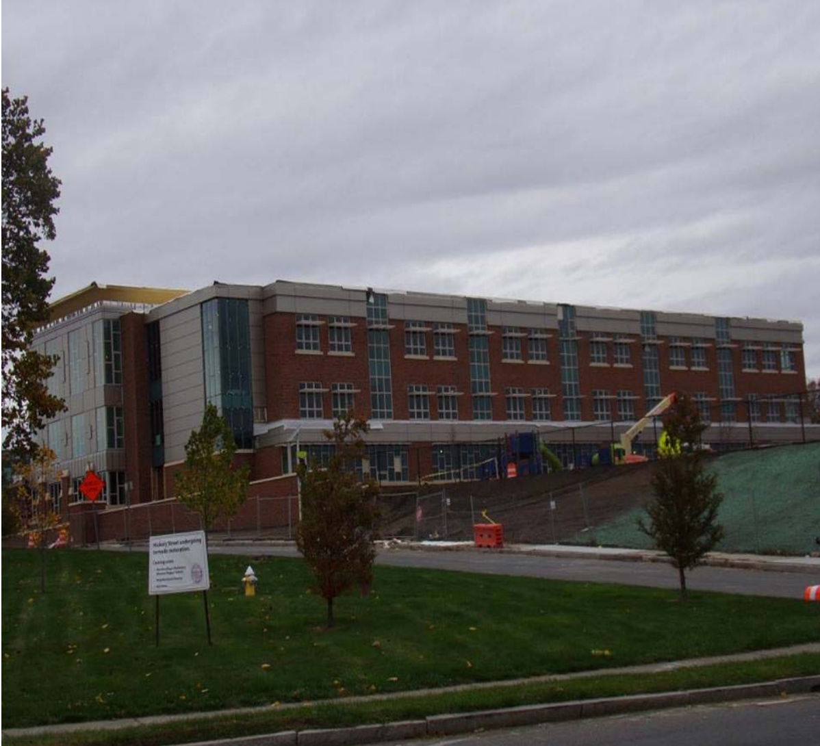
Construction of the new Elias Brookings Elementary School continues. To replace former school destroyed by the June 1, 2011 tornado.
