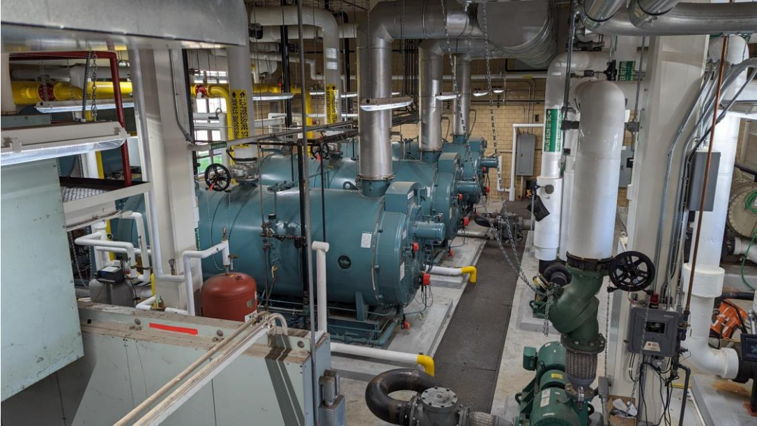
Sci-Tech Boiler Plant
