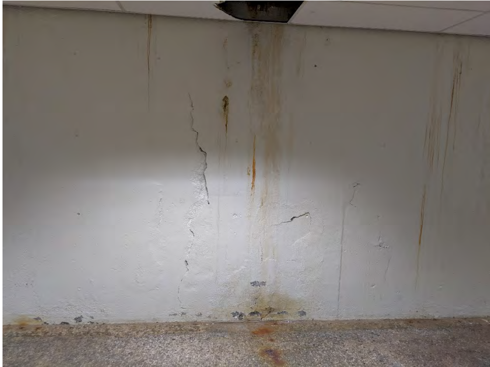
PHOTO 29: RUST STAINING BELOW CURB LINE UNDER BEAM 3 AT SOUTH ABUTMENT
