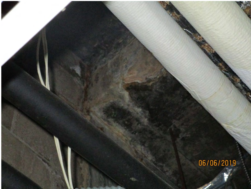
PHOTO 2: EFFLORESCENCE BELOW CONCRETE SLAB AT NORTHEAST CORNER OF BRIDGE
