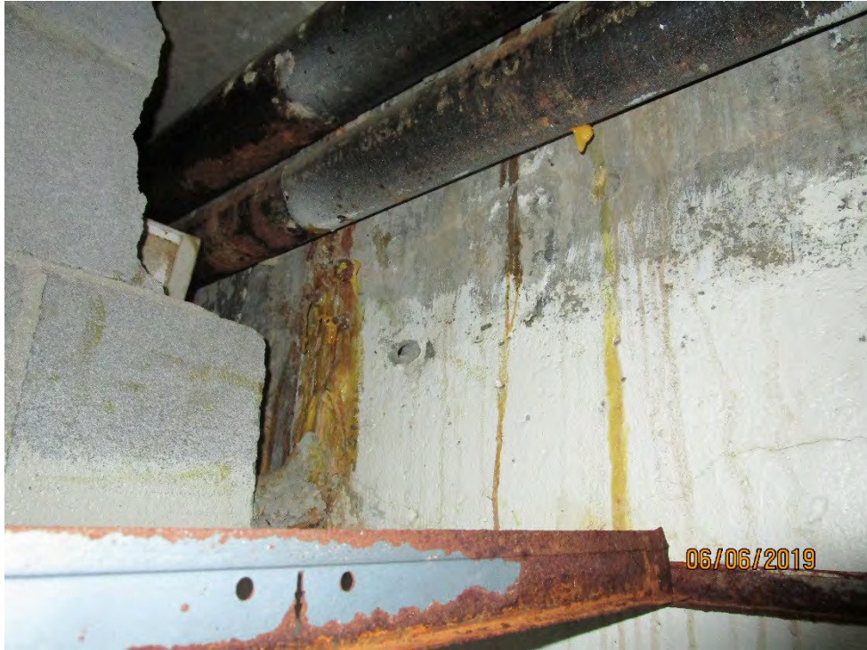
PHOTO 7: WATER INFILTRATION THROUGH NORTH ABUTMENT WALL BELOW BEAM 20
