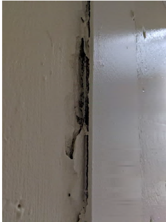
PHOTO 24: LAMINATED RUST AT SW CORNER OF SOUTH ABUTMENT EXPANSION JOINT
