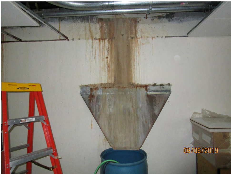
PHOTO 4: WATER INFILTRATION AT NORTH ABUTMENT BETWEEN BEAM 23 & EDGE BEAM 2
