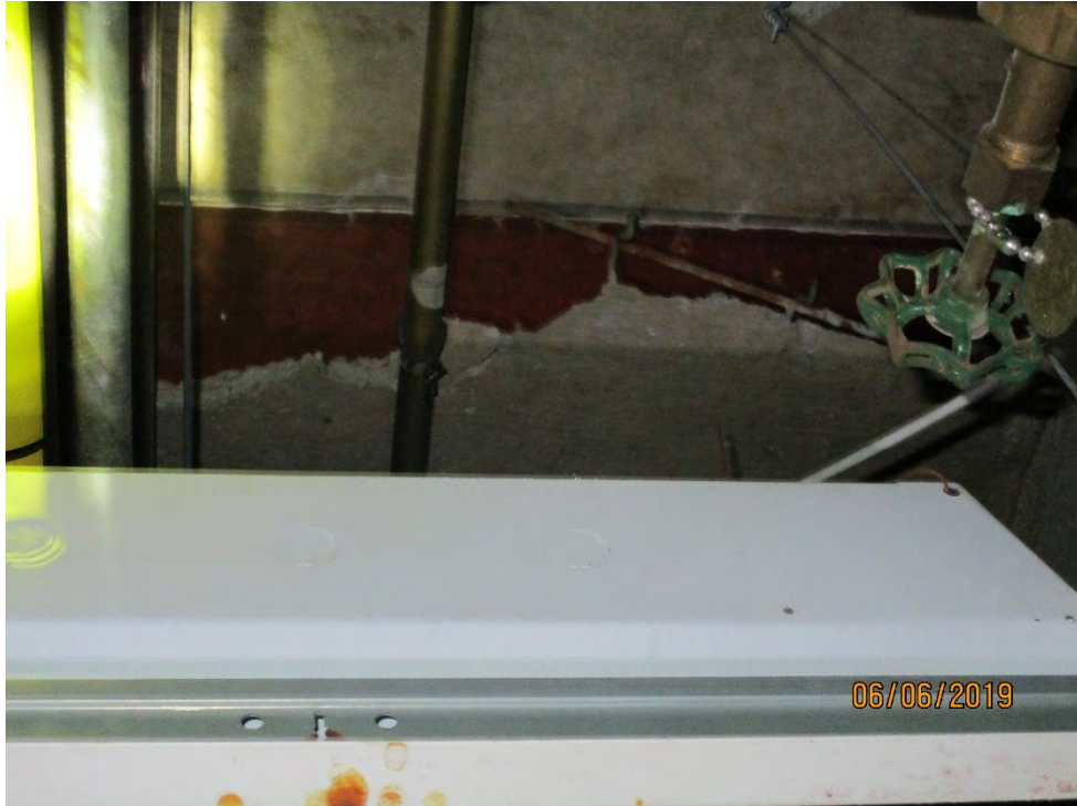
PHOTO 15: DELAMINATED CONCRETE AT UTILITY BAY BETWEEN BEAMS 2 AND 3
