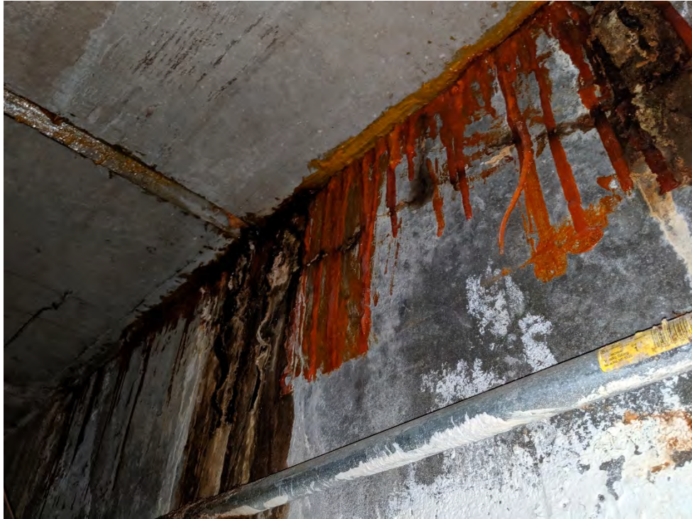
PHOTO 27: WATER INFILTRATION BETWEEN BEAMS 3 AND 4 AT SOUTH ABUTMENT
