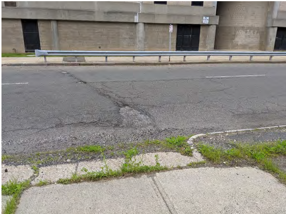
PHOTO 34: CRACKS IN PAVEMENT ON BIRNIE AVENUE OVER SOUTH ABUTMENT
