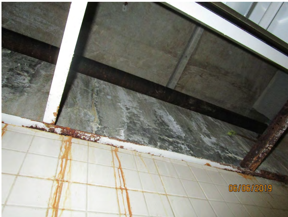
PHOTO 10: EFFLORESCENCE ON NORTH ABUTMENT BELOW BEAMS 14 AND 15
