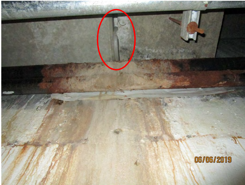
PHOTO 3: JOINT FAILURE AT NORTH ABUTMENT BETWEEN BEAM 23 & EDGE BEAM 2
