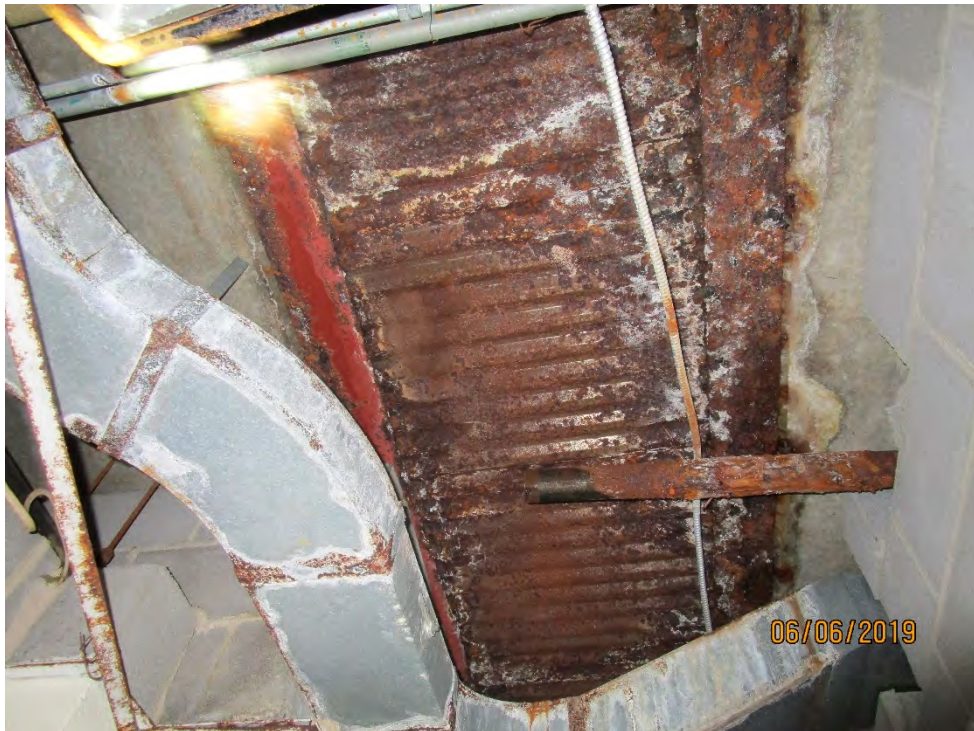
PHOTO 8: RUSTED ANGLES AND STAY-IN-PLACE FORM UNDER UTILITY BAY BETWEEN BEAMS 17 AND 18
