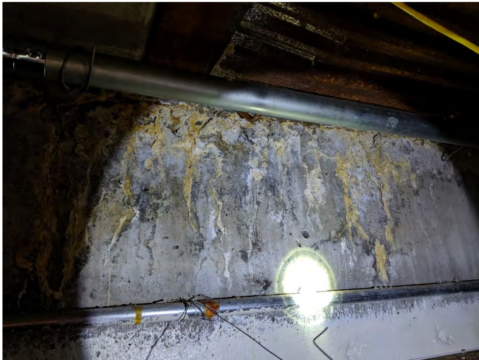
PHOTO 30: EFFLORESCENCE AT UTILITY BAY EAST OF BEAM 17 AT SOUTH ABUTMENT
