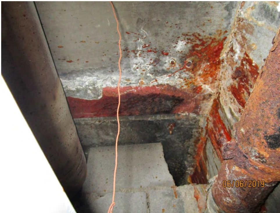
PHOTO 14: HEAVY RUST AT UTILITY BAY BETWEEN BEAMS 3 AND 4 AT NORTH ABUTMENT
