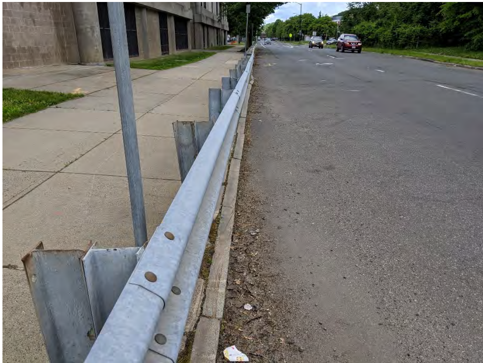
PHOTO 36: WEST SIDE OF BIRNIE AVENUE OVER BRIDGE FACING NORTH - NOTE EXISTING METAL GUIDERAIL
