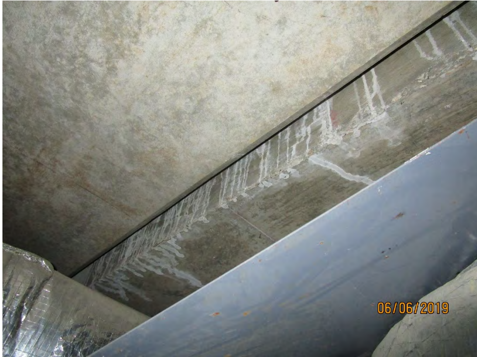
PHOTO 5: EVIDENCE OF LEAKAGE BETWEEN BEAM 23 AND EDGE BEAM 2
