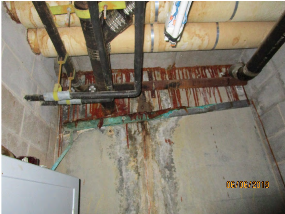
PHOTO 9: WATER INFILTRATION BETWEEN BEAMS 16 AND 17 AT BIRNIE AVENUE CURBLINE
