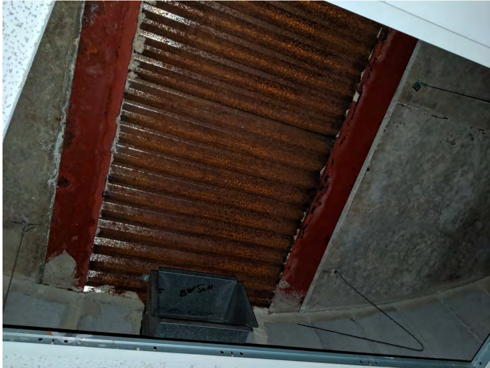
PHOTO 19: RUST AT UTILITY BAY BETWEEN BEAMS 17 AND 18
