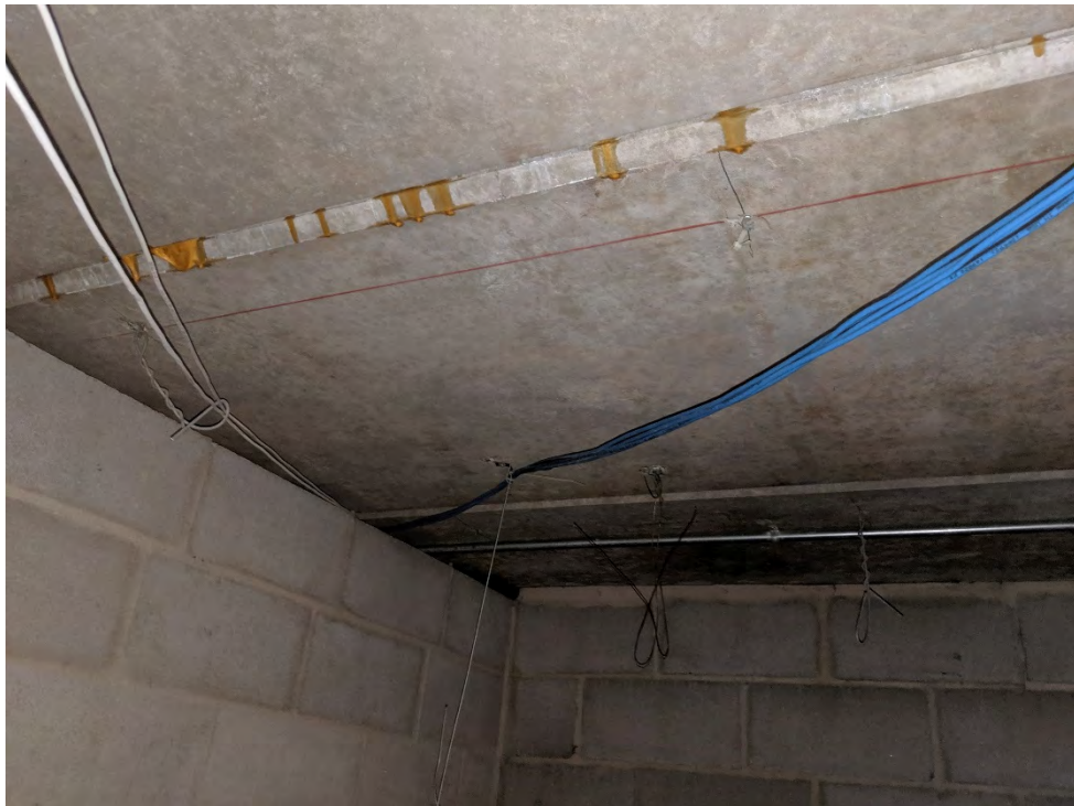
PHOTO 20: LIGHT LEAKAGE BETWEEN BEAM 21 AND 22 AT QUARTER POINT OF SPAN
