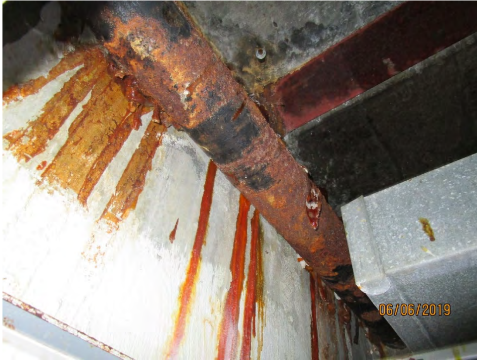
PHOTO 13: HEAVY RUST ON UTILITY CONDUIT UNDER BEAM 2 AT NORTH ABUTMENT
