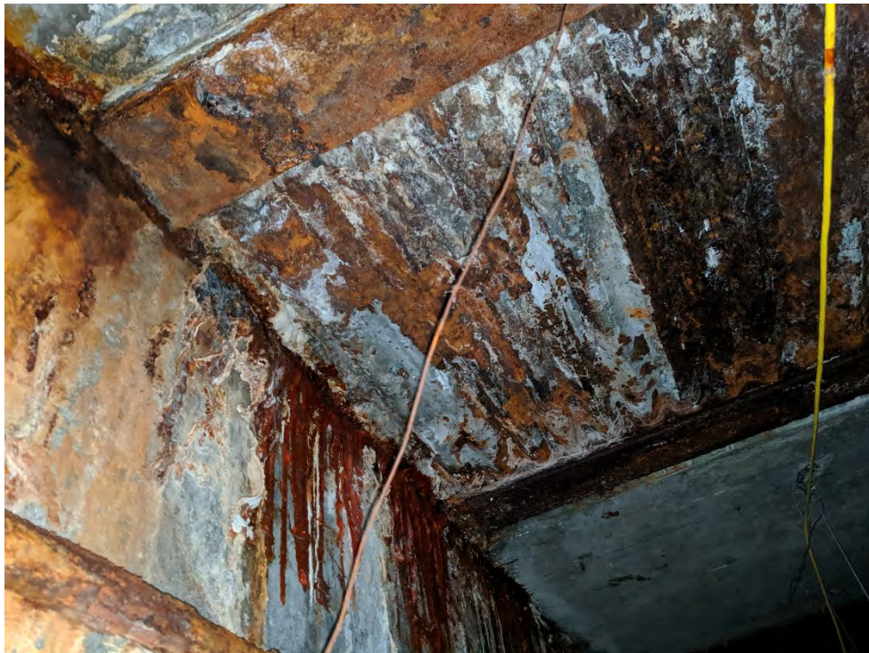
PHOTO 26: HEAVY RUST AND EFFLORESCENCE BETWEEN BEAMS 2 AND 3 AT SOUTH ABUTMENT
