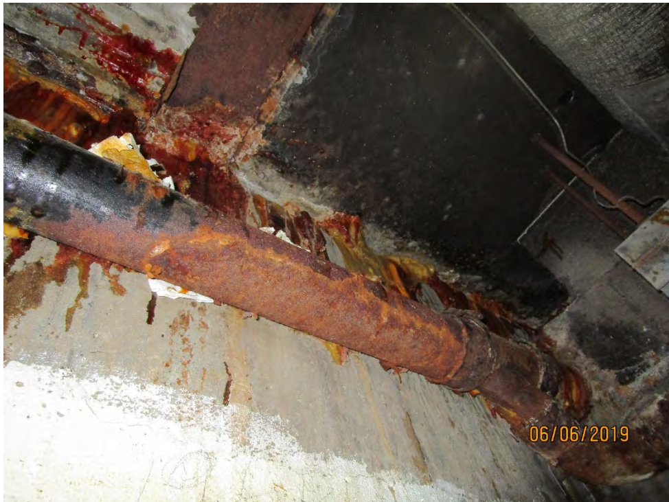
PHOTO 16: HEAVY RUST ON CONDUIT UNDER UTILITY BAY WEST OF BEAM 2
