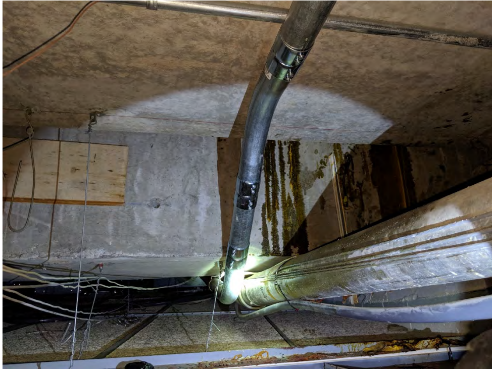
PHOTO 23: WATER INFILTRATION BETWEEN EDGE BEAM 1 AND PRESTRESSED BEAM 1
