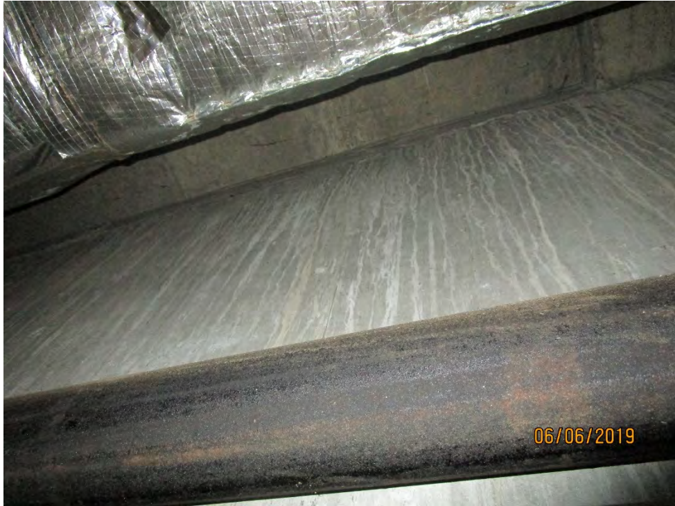
PHOTO 1: EVIDENCE OF WATER INFILTRATION AT NORTH ABUTMENT
