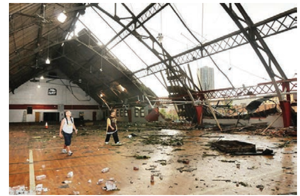
SECC Feildhouse, tornado damage
